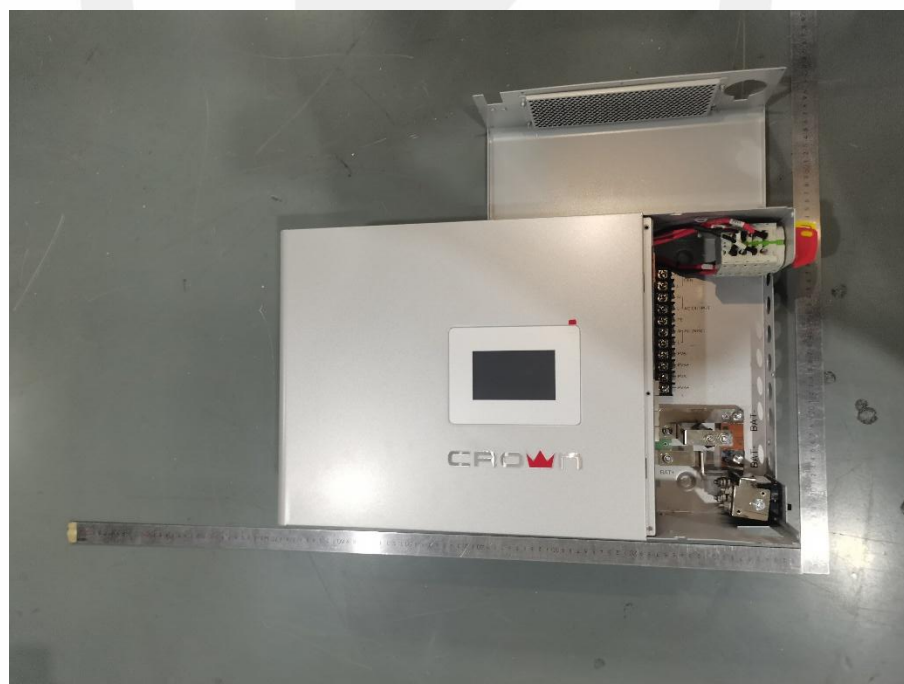
Fig. 8 -- Interior view (inverter)
